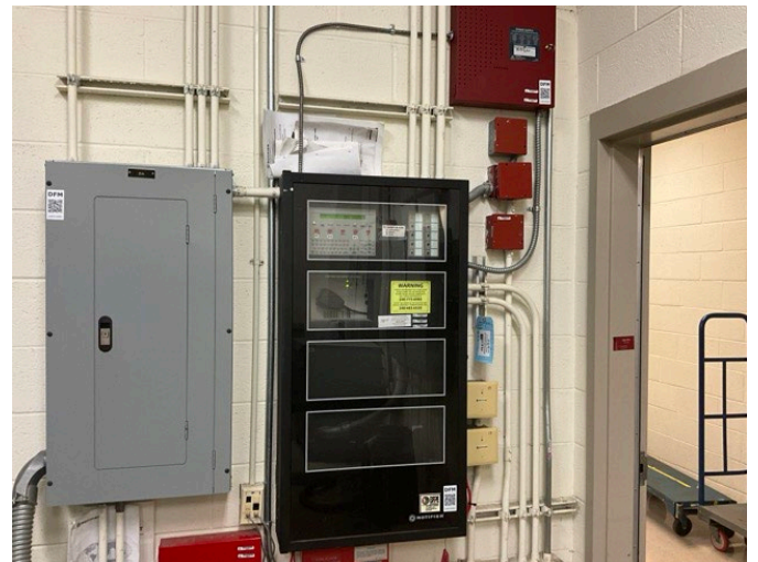
28 - FIRE ALARM PANEL
