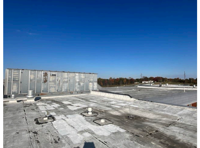
26 - ROOFTOP HVAC UNITS
