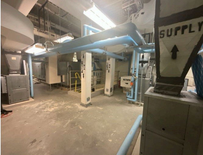
25 - SECONDARY MECHANICAL ROOM
