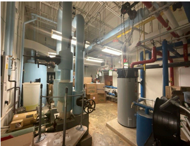
21 - MAIN MECHANICAL ROOM
