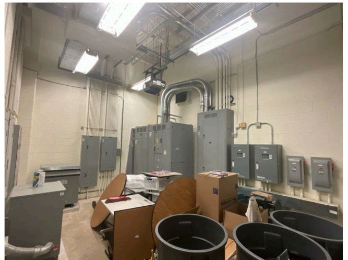
22 - MAIN ELECTRICAL ROOM
